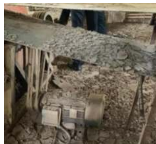
Conveyors and Motors
